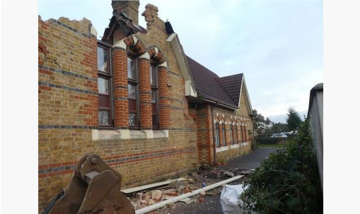
The Old School House being demolished, December 2020. Pictures by Cllr Angela Gunning.
